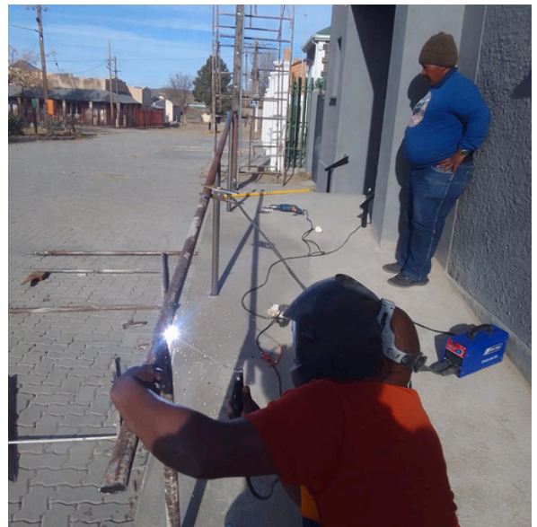
A safety rail being installed to provide assistance for people with wheelchairs.
